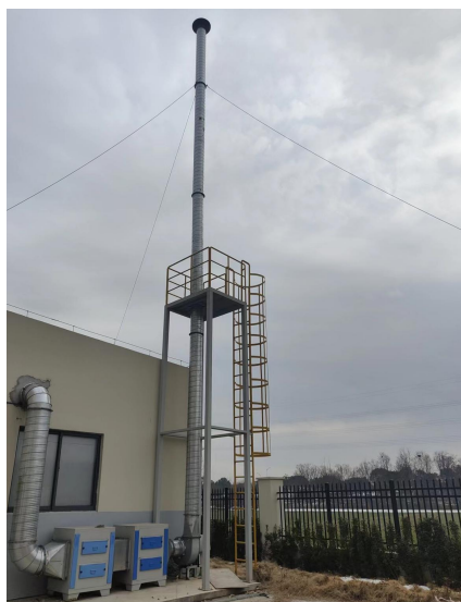
危废库废气密闭收集+二级活性炭吸附装置+DA004 排气筒
